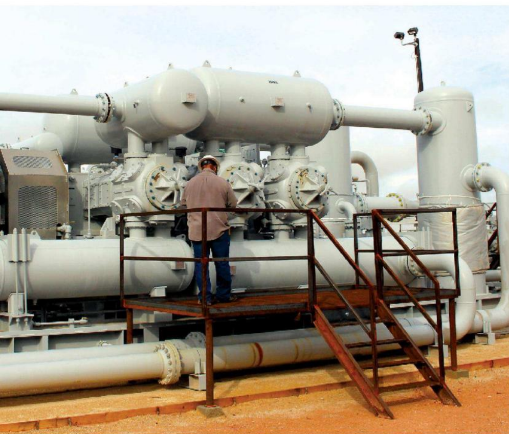
Monarch offers full turnkey solutions to help customers adopt electrification in their compression operations.
